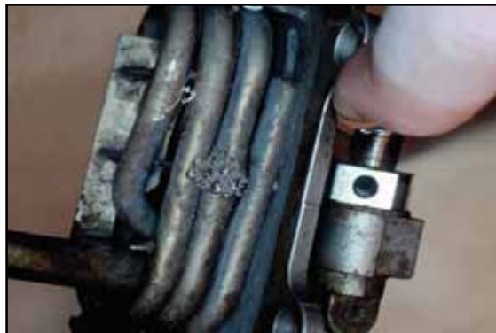
Photo No. 5: Sensing tube leak
