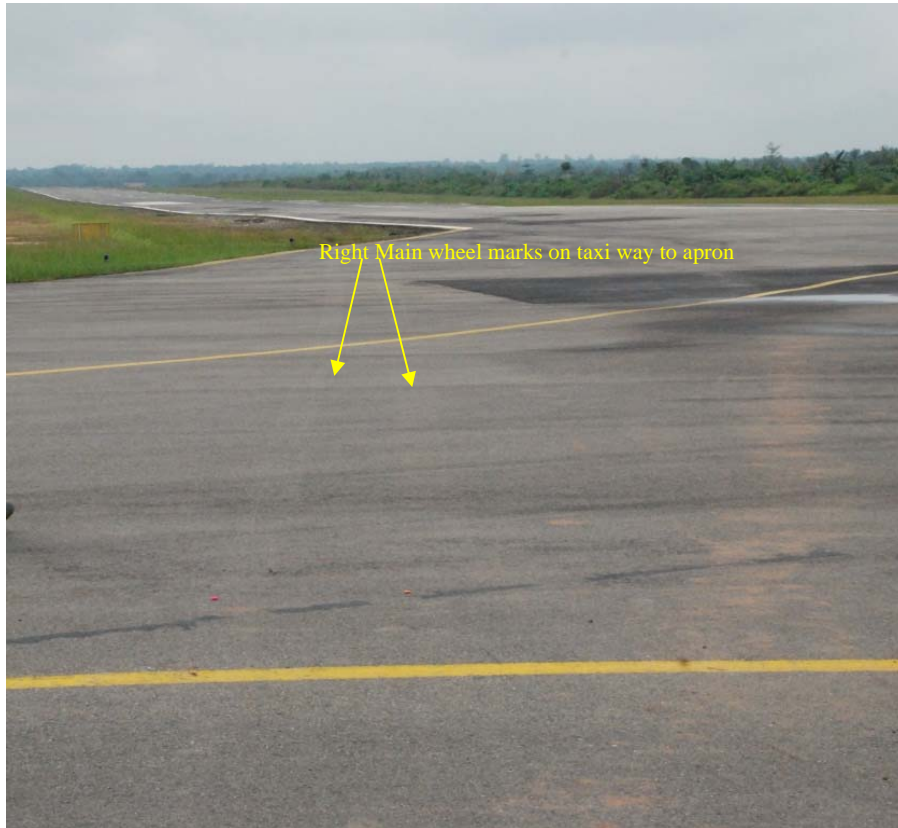
Figure 8: Main wheel marks on the taxiway to apron
